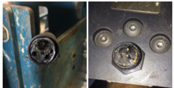
Magnet cord and magnet connector damaged due to overheating
