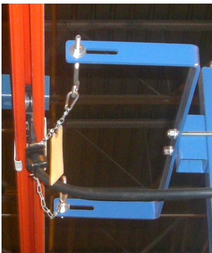
Improper alignment of Aeromotive energy rail and trolley
