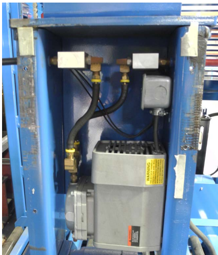
Cover/Stiffener Plates & Hardware missing
